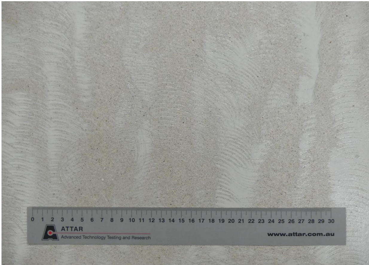
Figure 1: Dulux Avista Waterbased Sealer with Slip Reducing Additive applied to steel trowel finish concrete
